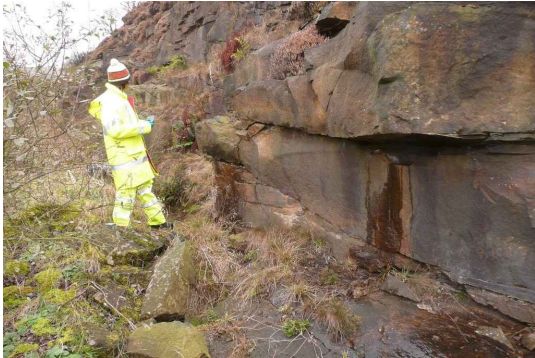
Water Seepage from a rock. 56
